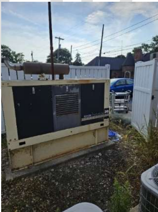
Generator at Station 38
