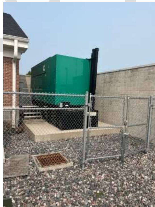
Generator at Station 39
